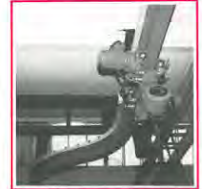
Electrification of hoist of a curved monorail.
