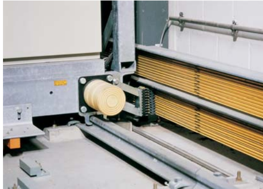
Conductor rail system in a high bay storage
