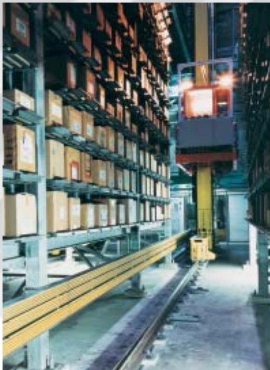
13 pole multipole conductor rail with double current collectors in the high bay storage of a warehouse.
