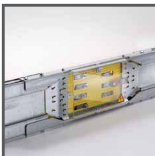
Additional power feed
